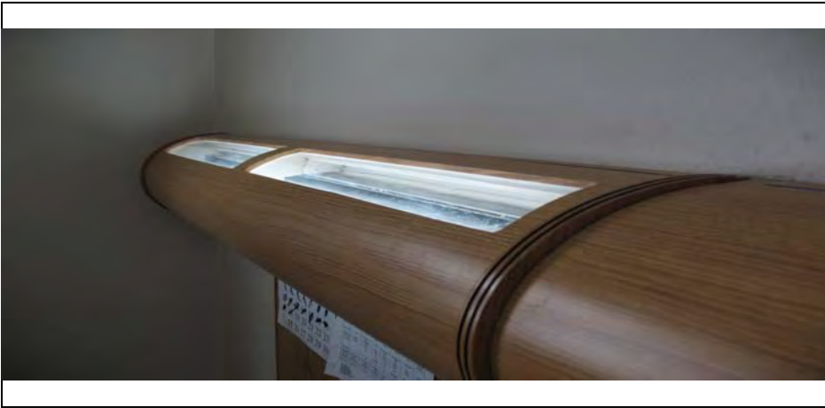
Figure 3.2.5.10: Over-bed Light Fixture
